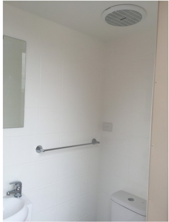
CEILING FAN. GPO. DOWN LIGHT
